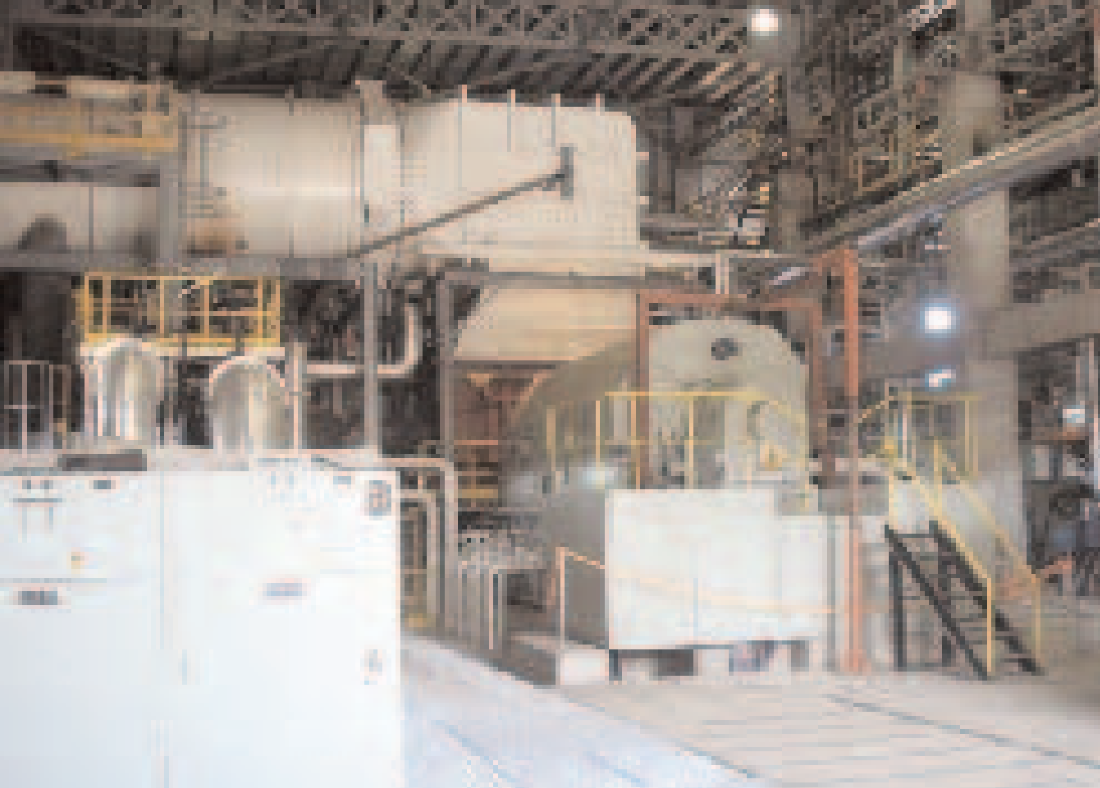
Steam turbine at Energia del Sur CCGT Conversion, Comodoro Rivadavia Plant, Patagonia, Argentina.
